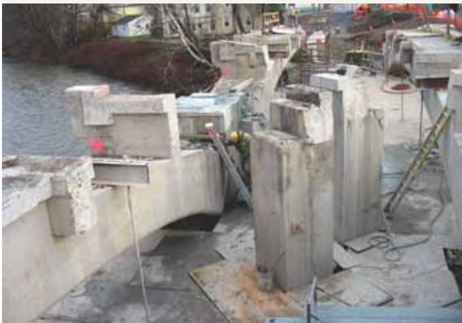
These were the components of the existing structure that were left in place after removal of the deck and floor beams.
