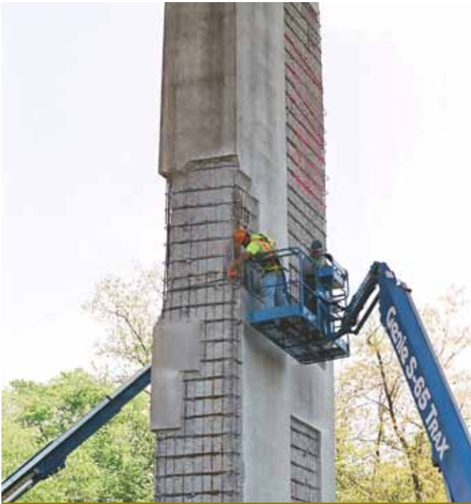
Shotcrete was used to repair the 86 piers on the 7122-ft-long Abraham Lincoln Memorial Bridge in LaSalle, Ill., the longest bridge in the state. Using shotcrete ensured contractors could visually check encapsulation of the reinforcing steel.
