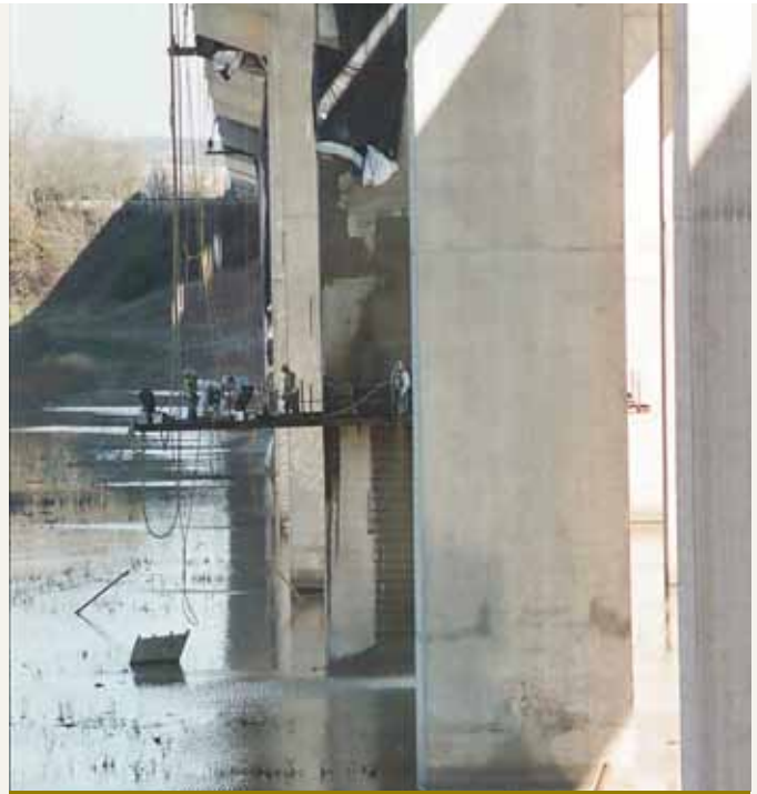
All work was completed from overhead, which provided less risk due to the ability to feed air and water hoses over the side rather than handling formwork.
