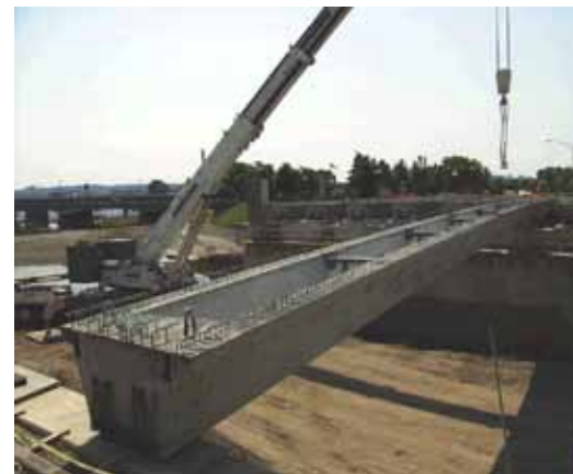
The Edwin C. Moses Boulevard Bridge features 48-in.-deep precast, prestressed concrete U-beams, the first U-beams to be used in Ohio. Photo: City of Dayton, Ohio.
