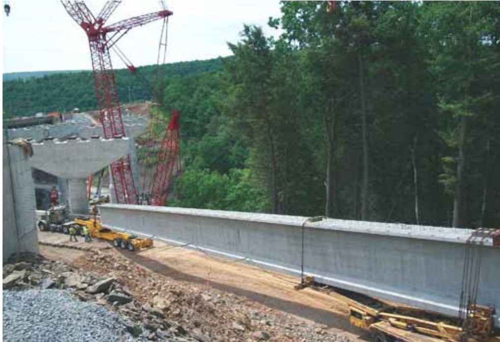
Fifty precast, prestressed concrete beams with lengths greater than 163 ft were required for the bridges and delivered to the site and erected without extraordinary provisions.
