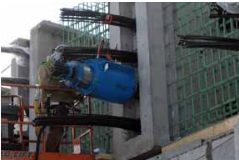
After splices were cast and cured, each of five tendons was pulled to approximately 960 kips. Photo: VHB—Vanasse Hangen Brustlin Inc.
