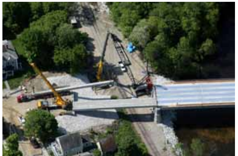
Span 3 box beams were erected through a sequence of carefully choreographed crane movements. In this photo, one crane passes the end of a box beam to another crane for final placement. Photo: VHB—Vanasse Hangen Brustlin Inc.
