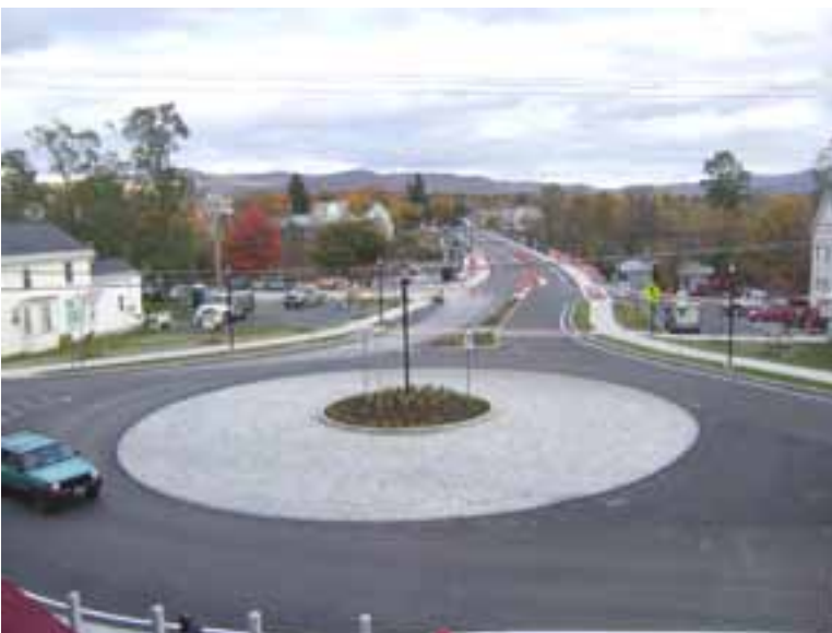
A newly constructed roundabout compliments the project with the nearly completed bridge in the background. Photo: VHB—Vanasse Hangen Brustlin Inc.
