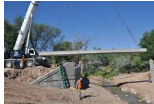
Construction on the D Road Bridge over the Redlands Water and Power Canal took place during the winter to prevent interruption to irrigation water. Prestressed concrete girders were used on this bridge as well.
