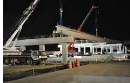
Girders for the 29 Road Bridge were placed at night to limit disruption to daytime traffic on I-70B.
