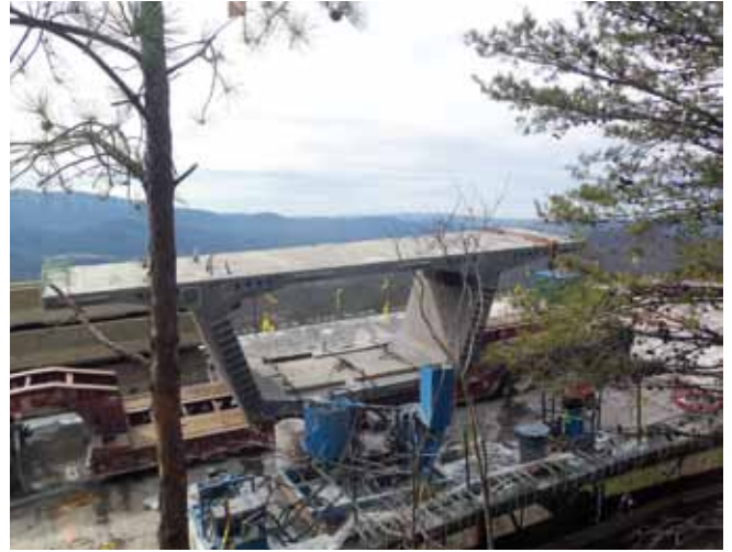
The segments were trucked 40 miles from the casting yard to the bridge site.
