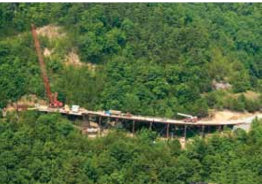
The temporary work trestle construction advances from right to left. A secondary crane provides access for foundations and pier construction.
