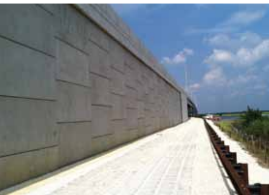
MSE retaining wall and articulated concrete block mattresses were used as an access road.
