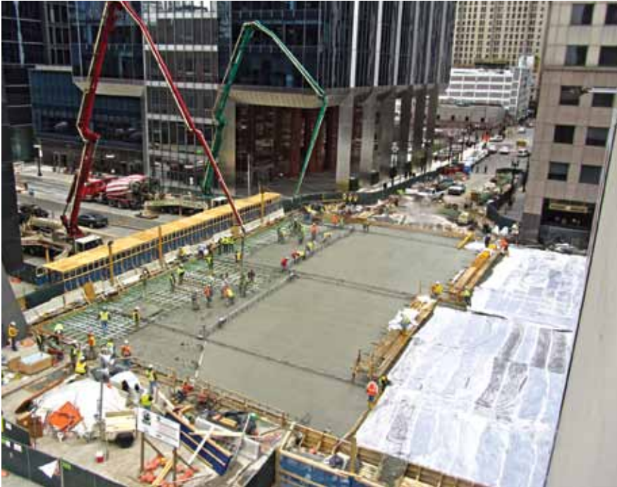
View of first placement of concrete for the deck. Photo: McHugh Construction.
