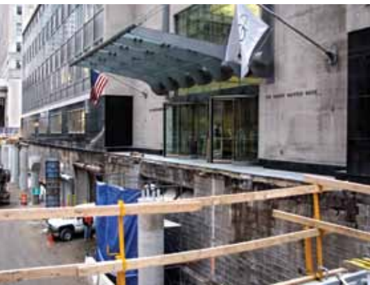
Example of the close proximity of the adjacent buildings to the viaduct. Photo: Alfred Benesch and Company.
