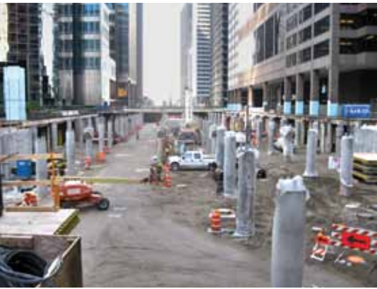
Looking south along Wacker Drive with the new columns in place and waiting for the decking. Photo: Alfred Benesch and Company.
