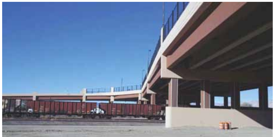
The completed 29 Road Bridge and the intersection of the I-70B Ramp on the left. Photo: Paul Jagim, City of Grand Junction, Colo.
