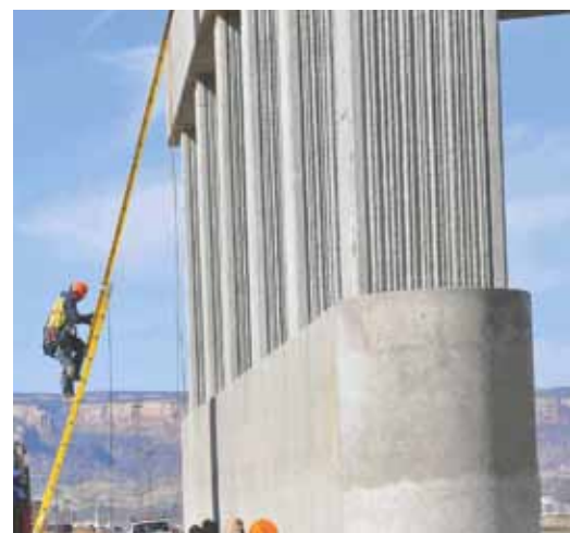
The cast-in-place pier columns are shown with crash protection wall and striated surface that will be stained. Photo: Kristin Winn, City of Grand Junction, Colo.
