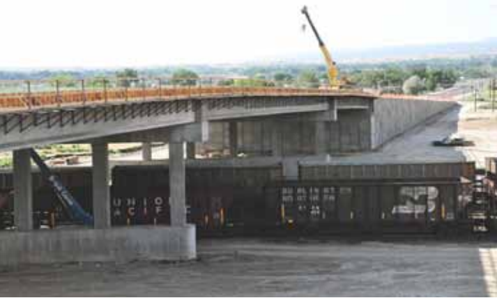
Construction of the spliced-girder unit over the UPRR showing the MSE approach retaining walls. Photo: Kristin Winn, City of Grand Junction, Colo.
