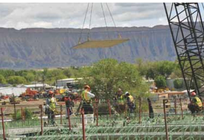
A 3½-in.-thick, precast, prestressed concrete, stay-in-place deck panel form being lowered to the bridge during installation. Photo: Kristin Winn, City of Grand Junction, Colo.
