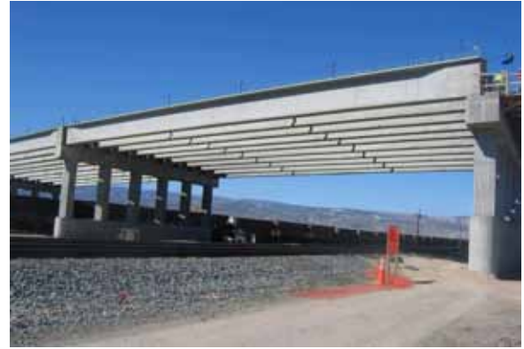
Post-tensioning of the three-span, spliced-girder unit over the UPRR tracks. Photo: Jacobs Engineering Group Inc.
