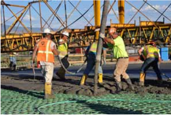
Placement of concrete for the deck on the partial-depth deck panels. Epoxy-coated reinforcement was specified to extend deck durability. Photo: Kristin Winn, City of Grand Junction, Colo.
