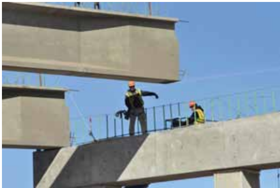
Erection of the spliced girders showing the flared end to accommodate post-tensioning anchors. Photo: Kristin Winn, City of Grand Junction, Colo.
