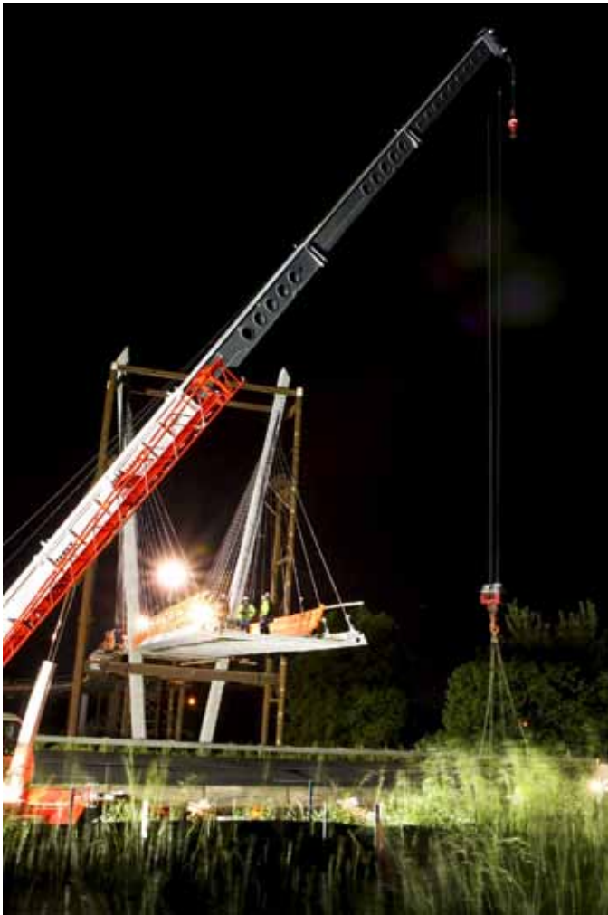
Using a stay supported cantilever system and precast concrete deck panels, construction crews were able to extend the bridge deck in segments over the highway.
