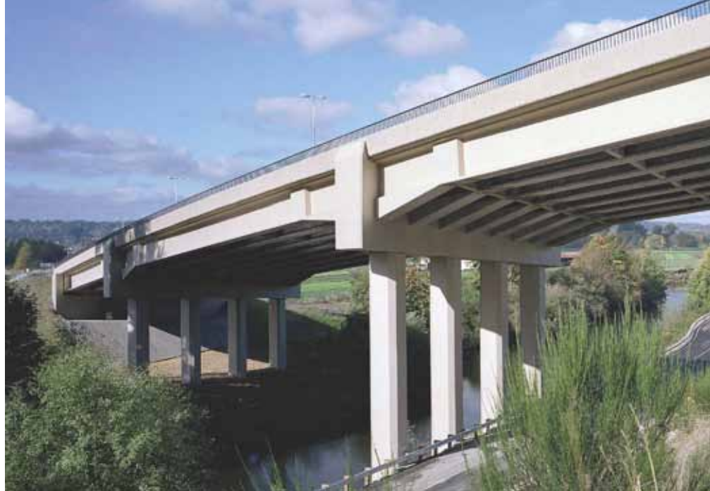
The Don E. Wickstrom Bridge over the Green River in Kent, Wash., features fully continuous, post-tensioned spans and integral piers. Photo: BergerABAM.
