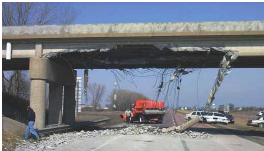
An accident caused by an over height load on I-29 in Iowa, resulted in the destruction of all bottom flanges of this precast, prestressed concrete I-girder bridge without its collapse, illustrating the redundancy in these concrete structures. Photo: Iowa Department of Transportation.
