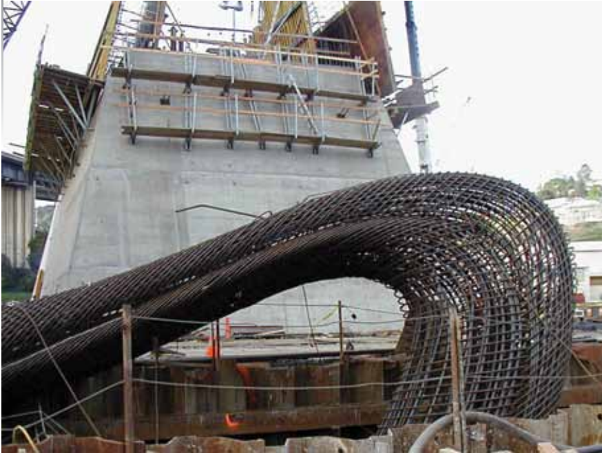
Close-up of a collapsed cage on a jobsite. All photos and drawings: University of Nevada in Reno.
