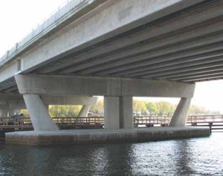
The new Route 70 Bridge over Manasquan River in New Jersey. Photo: Aurora & Associates.
