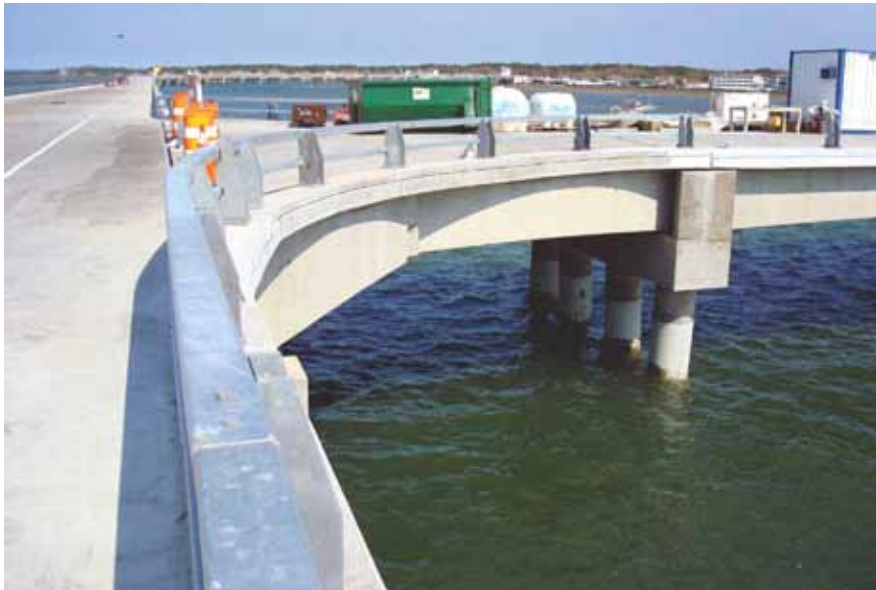
The diagonal dapped beam spans between the mainline pier and a bracket on the fascia beam of the connector bridge. Photo: Virginia Department of Transportation.
