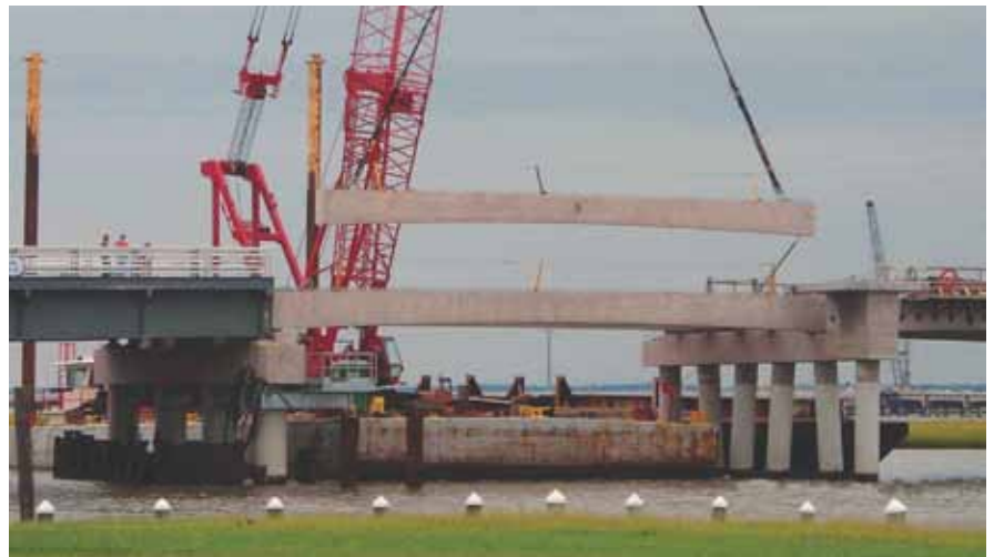
Fascia beam being erected for the new Chincoteague Island Bridge. Photo: Hardesty & Hanover.
