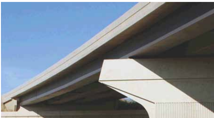
Arbor Road Bridge over I-80 in Lincoln, Neb., used curved precast concrete box girders.
