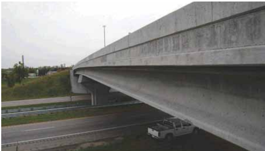
Grand Island Bridge over I-80 utilizes threaded 150 ksi reinforcing-bar connections for full continuity of dead load and live load over the support.
