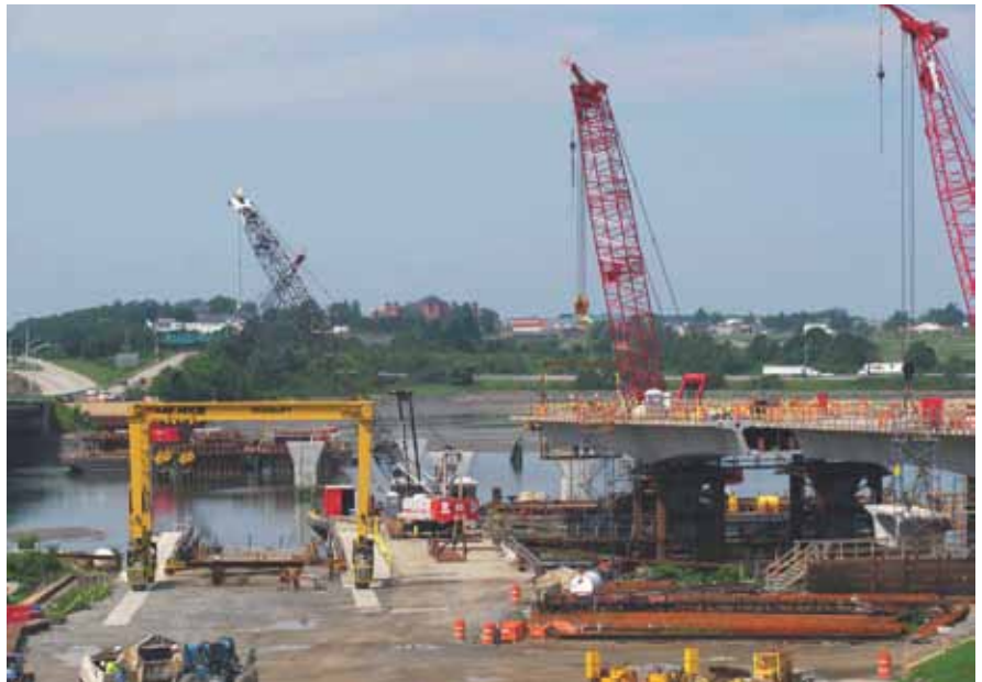
Segments were carried to temporary docks and loaded on barges to be delivered to the cantilever tips. Photo: Reed & Reed Inc.
