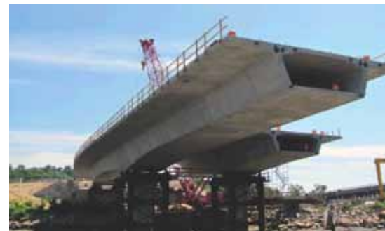
Segments cantilever out from Pier 6 at the north end of the bridge. Photo: Reed & Reed Inc.
