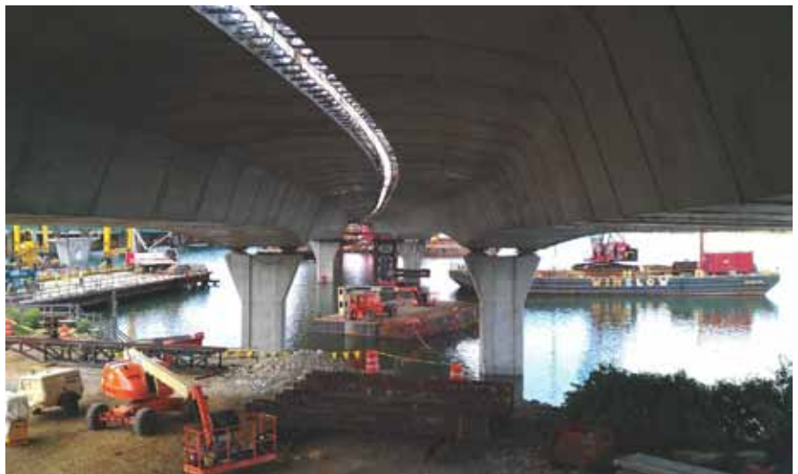
Once the two structures were erected, a cast-in-place closure strip joined the two halves, creating a continuous deck surface. Photo: Reed & Reed Inc.
