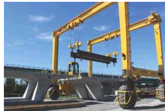
In the yard, segments were shuttled with a straddle lift. Photo: Reed & Reed Inc.
