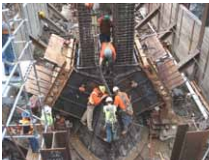
Casting of the reinforcement-congested bent 3 shaft cap/arch rib/column joint with special high-slump 6.0 ksi concrete.
