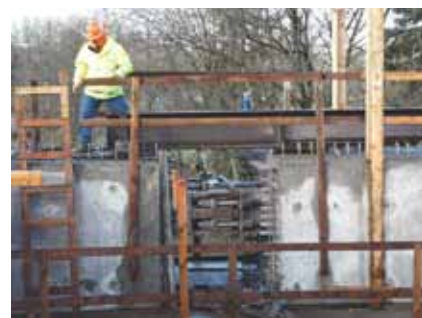
Span 2 ribs become self-supporting after crown jacking. Weight of each rib is carried by eight, 2.5-in. diameter, 150 ksi post-tensioning rods, two of which are visible at the side of the jacking frame.
