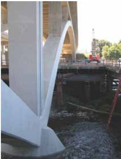
Finished view of bent 3 shaft cap/arch rib/column joint in foreground, with floor system visible above. At far end of rib, a solid soffit of post-tensioned box girder spans adjoins arch span.
