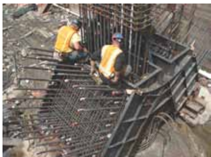
Placing column bars through rib reinforcement in bent 3 joint. Shaft cap skin reinforcement remains to be placed along with remainder of steel forms.
