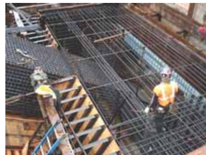
Shaft and rib reinforcement extending into partially-completed bent 2 shaft cap reinforcement cage. Column bars are not yet placed.
