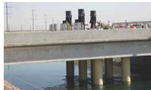
All six pump cans extend below deck into the canal and three pump-motor assemblies are mounted above.
