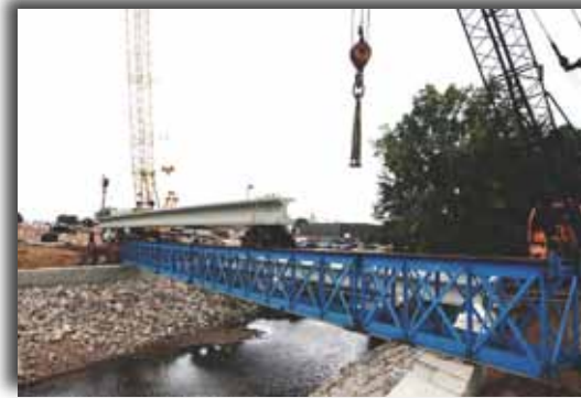
The leading end of the beam was mounted on a trolley on the beam launcher. The delivery truck pushed it across the Fond du Lac River until it could be reached by the near crane. Together, the two cranes lifted and set the beam in place. Photo: Steve Hinkley, retired, city of Fond du Lac, Wis.
