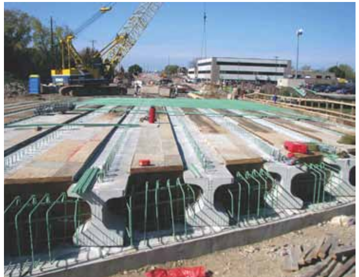
The 8-in.-thick composite deck is shown being formed on the Wisconsin 36W ® beams. Epoxy-coated reinforcement was used to help ensure a long service life. Photo: Jim Lucht, AECOM.
