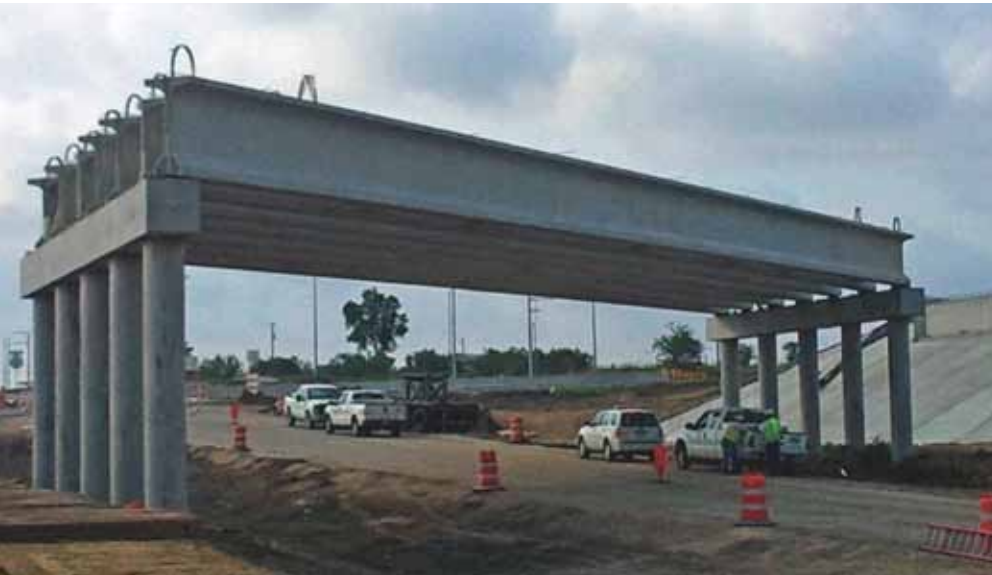
Fourteen precast concrete Type VI modified beams that were 164 ft 8 in. long were the longest ever used in the state. All photos: Heldenfels Enterprises Inc.
