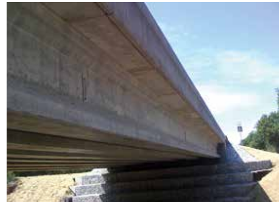
The underside view of the Farm-to-Market Road 1885 Bridge over Rock Creek near Cool, Tex., shows the use of the precast, prestressed concrete overhang panel system.
