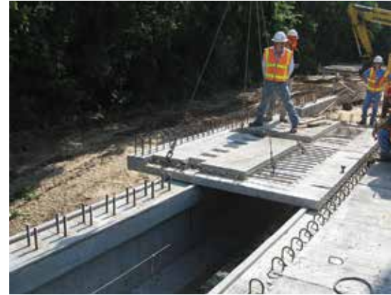
Placing and aligning precast, prestressed concrete overhang panels used on the Farm-to-Market Road 1885 Bridge over Rock Creek.
