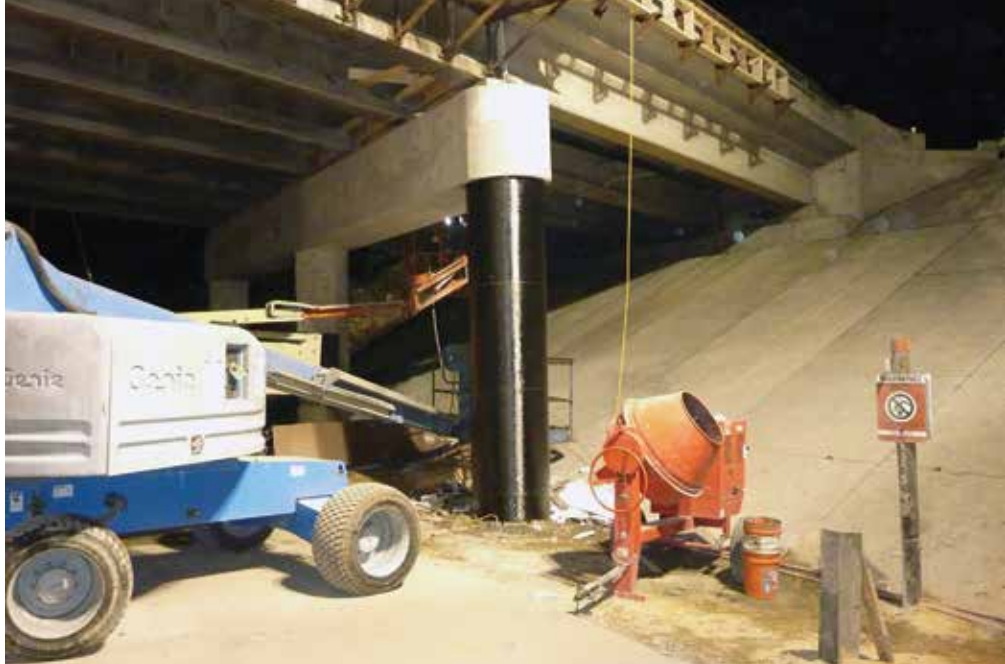
An example of column repairs for the Florida Turnpike over the SR 561 Bridge.
