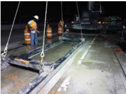
This photo shows sawing of the deck panel and attaching the lifting frame to the section for removal of existing deck during a nighttime replacement operation.
