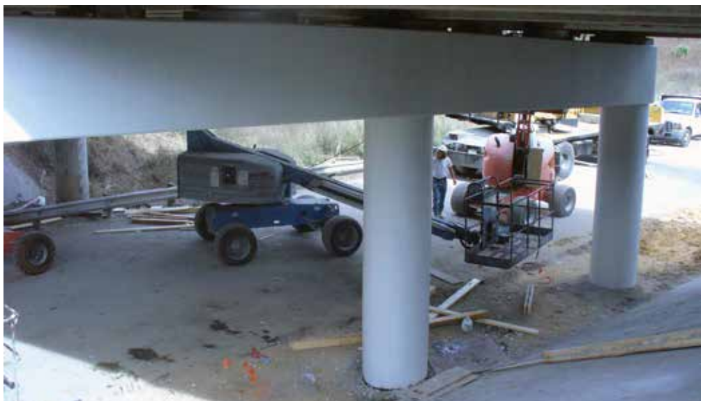
Another view of the repaired columns and pier caps that were part of the rehabilitation project for the Florida Turnpike over the SR 561 Bridge.
