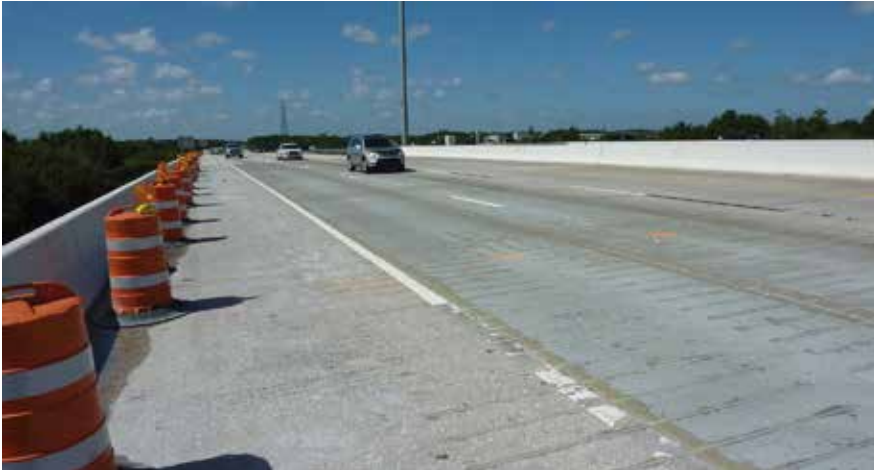
The completed full-depth deck replacement for the Highway I-75 project near Tampa utilizing sawed in carbon reinforcement connections. All photos: SDR Engineering Consultants Inc.
