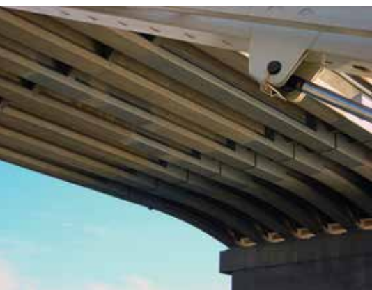
Completed carbon-fiber reinforced polymer repairs of the drop-in span and cantilever spans.
