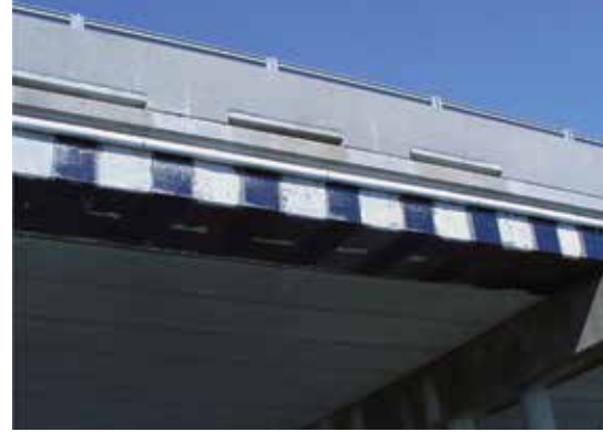
Fascia girder of adjacent box girder overpass repaired with carbon-fiber reinforced polymer.
