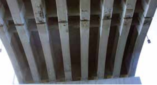
Deteriorated drop-in span hinge location before repair.
