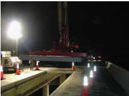
The new full-depth deck panel is ready for installation for the Highway I-75 project near Tampa.
