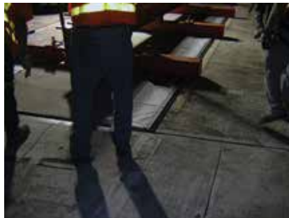
The panel is aligned in place and shimmed 1.4 in. higher than the existing deck to allow for future grinding, ensuring a smooth travelling surface.
