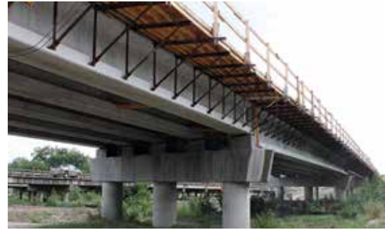
U.S. Highway 75 reconstruction project in McKinney, Tex. shows TX46 and TX62 girders spanning the East Fork of the Trinity River.
