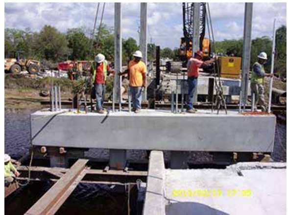
Bent erection and leveling — precast pile cap being checked for final grade before release from crane.
