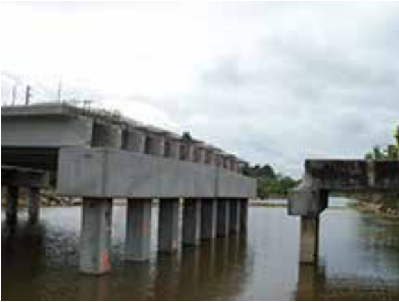
Contrast between new bridge on the left and existing bridge on the right.
