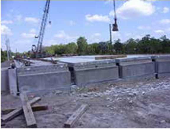
Looking east — west end of bridge — end diaphragms cast by second pour at the fabricator. All photos: Collier County, Fla.
