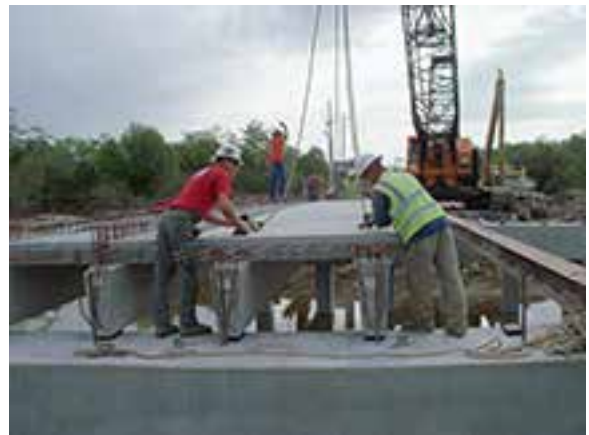
Setting the beams in place at intermediate bents No. 1&2 – releasing the lifting clamps after beam is in place.
