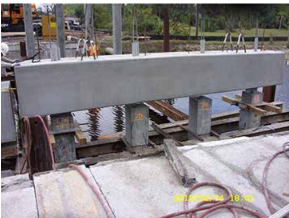
Setting bents — setting the pile cap on piles at intermediate bent No. 2.
