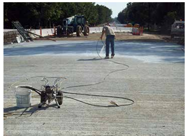
On the third day, the water cure was stopped, a heavy application of compound was applied, and traffic started to use the bridge.
