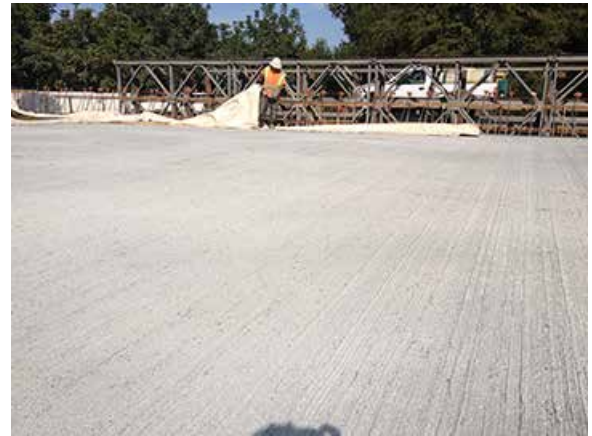
The high-performance concrete deck was cured using pigmented Type 2 compound and water.
