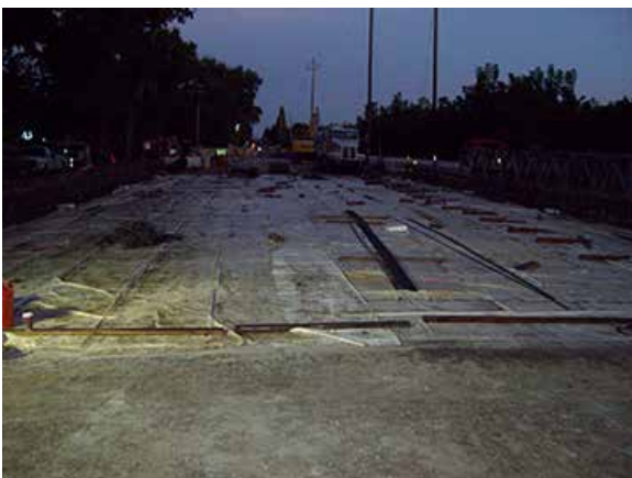
The high-performance concrete deck was water cured for three days – two-day strength was 3.2 ksi.
