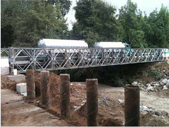
Pre-driven, cast-in-steel-shell concrete piles excavated after old bridge demolished. Traffic diversion took place on a rented bridge. All photos: Caltrans.
