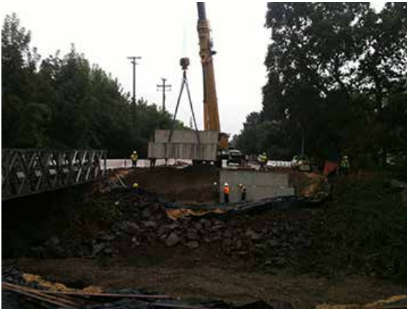
Precast concrete abutments were placed in single stage; no roadway shoring was required due to the value engineering cost-reducing proposal from the contractor.
