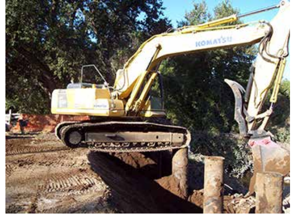
Cast-in-steel-shell concrete piles were ordered 9-ft longer and driven out of sequence to reduce impacts. They were excavated after traffic was detoured.
