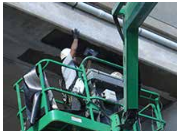
Carbon fiber reinforced polymer was wrapped around columns and pier caps as part of the rehabilitation project for the Florida Turnpike over the SR 561 Bridge.
