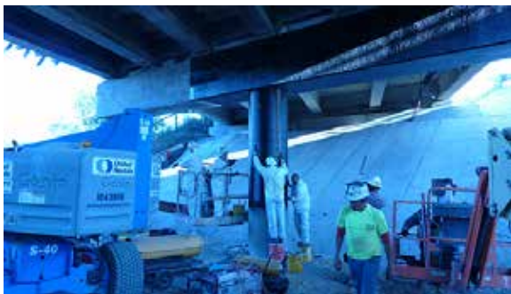
Workers apply carbon fiber reinforced polymer to columns and pier caps as part of the rehabilitation project for the Florida Turnpike over the SR 561 Bridge.
