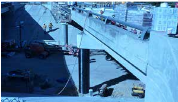
Another view of the carbon fiber reinforced polymer column repairs for the Florida Turnpike over the SR 561 Bridge.
