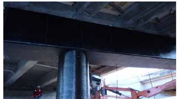
Carbon fiber reinforced polymer was wrapped around columns and pier caps as part of the rehabilitation project for the Florida Turnpike over the SR 561 Bridge.
