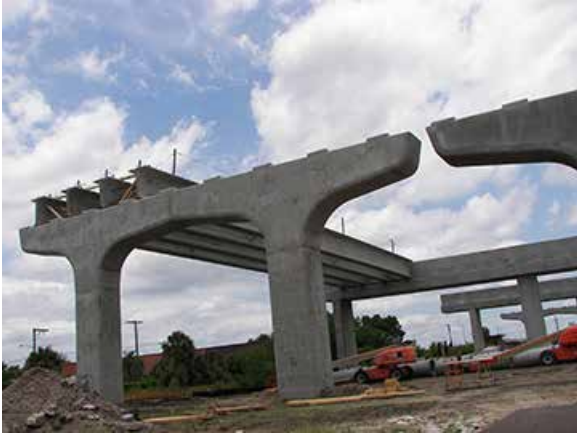
This photo shows Florida bulb-tee girders erected between double hammerhead and inverted-tee caps. All photos: Florida Department of Transportation.
