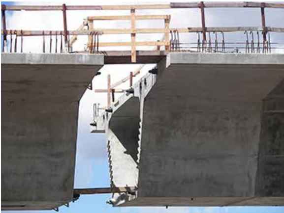
The gap between the precast segments will be filled by a cast-in-place segment.
