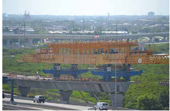
The massive overhead trussed gantry lifts segments into place along the Selmon Expressway, in Tampa, Fla.
