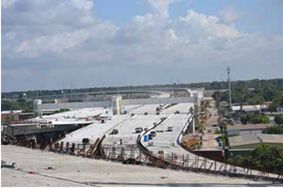
A look at the toll gantry from atop one of the segmental bridges.
