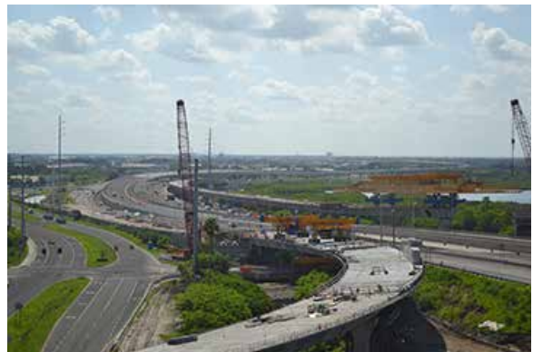
Segmental bridge construction along the Selmon Expressway (right) using an overhead trussed gantry and between the Selmon and State Road 60 using segment lifters.
