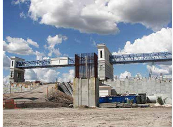
The toll gantry work site shows the huge amount of fill needed as the MSE walls are constructed to hold back the soil. Decorative panel installation is underway on the gantry and the towers.
