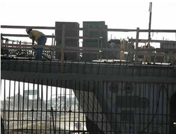
A worker is high above busy Interstate 4 morning traffic on a pier segment.
