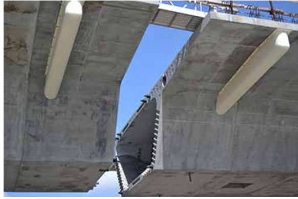
The gap between the precast segments will be filled by a cast-in-place segment.
