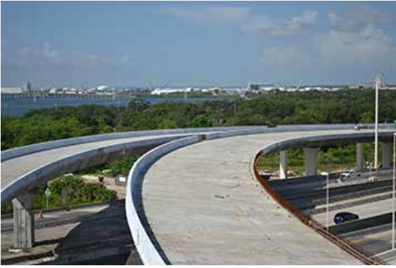
Nearly completed segmental bridges crossing the Selmon Expressway that will serve as the “truck only” ramps between the Port of Tampa and Interstate 4.
