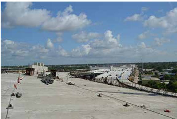
Taken from one of the highest spans in the project, the main corridor is taking shape between State Road 60 and Interstate 4 (top of photo). The structure spanning all lanes in the middle of the photo is the tolling gantry.
