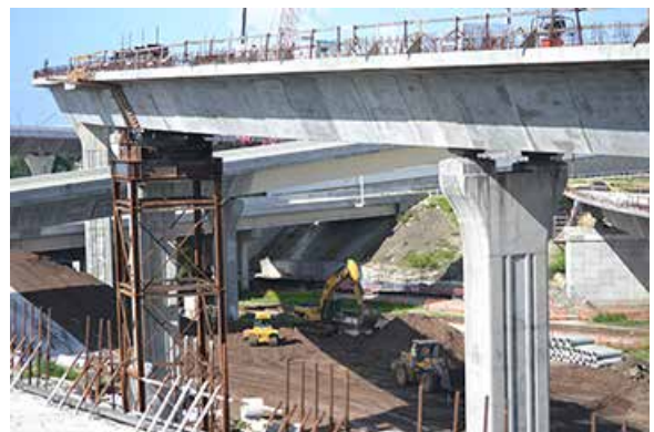
Several levels of segmental bridges cross in the heart of the project next to the Selmon Expressway.
