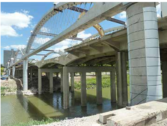
The arches were erected on both sides of the existing bridge to minimize closure times. Photo: TxDOT.
