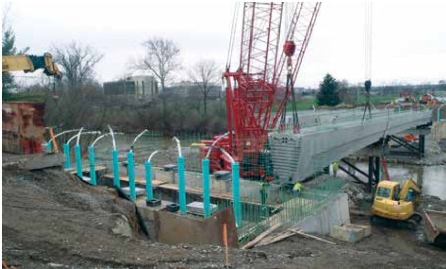
Erection of the precast concrete segments and view of the abutment tie-downs.
