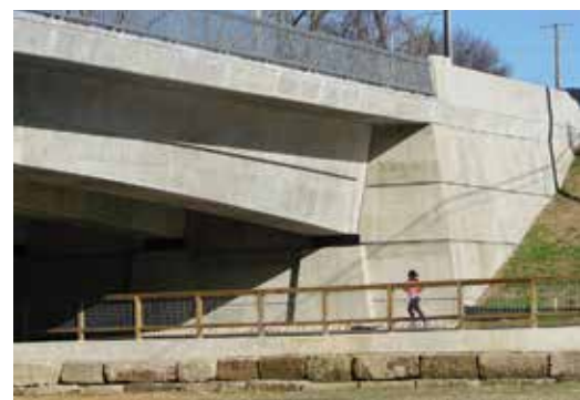
Aesthetic treatments to the substructure units. The end span is hidden behind the abutment.
