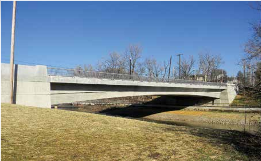
Bridge profile (east end). The Dodridge Street Bridge has a main span of 200 ft and two hidden end spans of 20 ft 6 in. All photos: E.L. Robinson Engineering.
