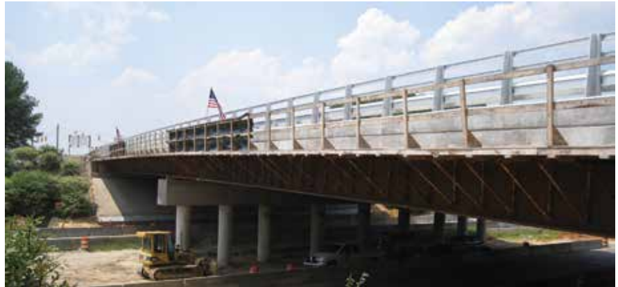
Lightweight concrete was used in the deck of the Morganton Bridge to reduce deck weight so that the existing columns and foundations could be retained. Photo: Carolina Stalite Co.
