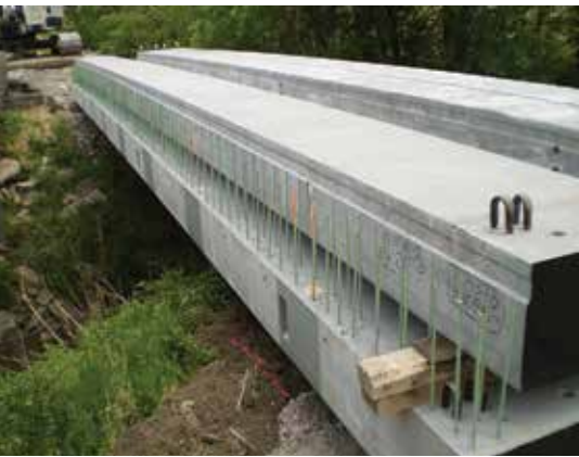
Stacking and storing bridge beams on site prior to construction provided added efficiency.
