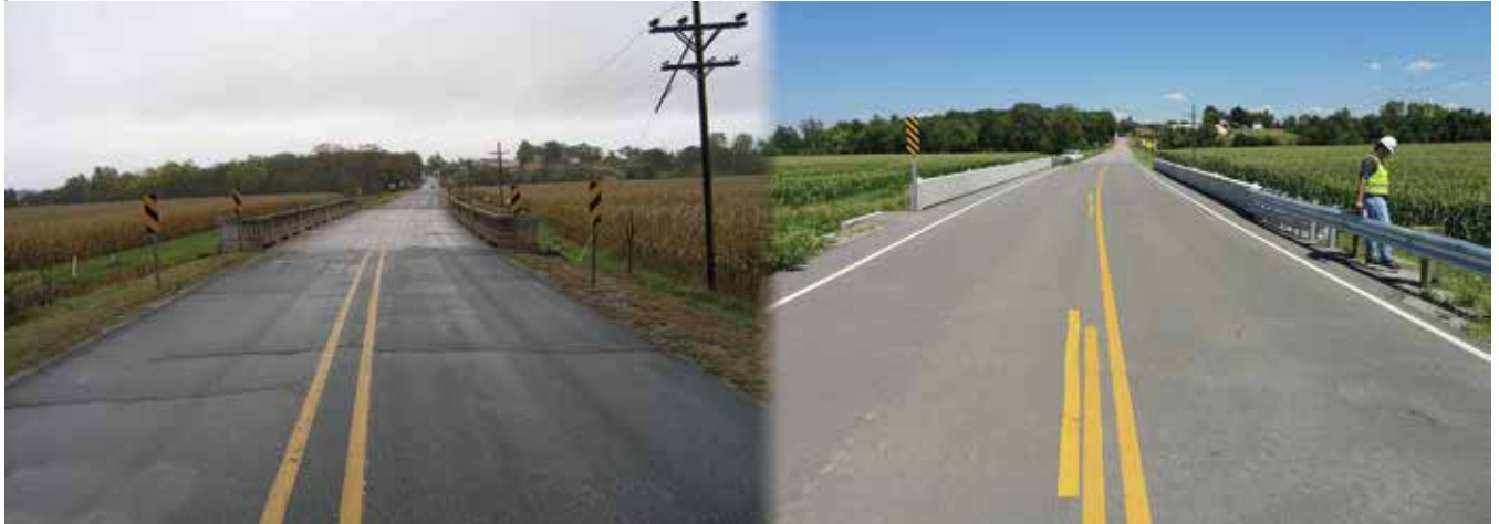
Old bridge before construction (left) and new bridge after construction (right), Andrew County Route 98. All photos: MoDOT.
