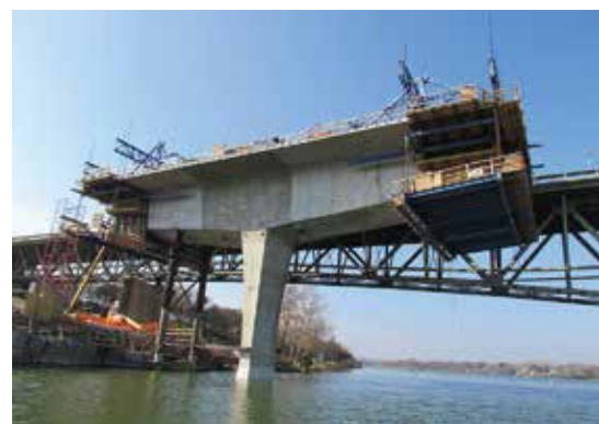
Partial cantilever with temporary stability support to the left of the pier.
