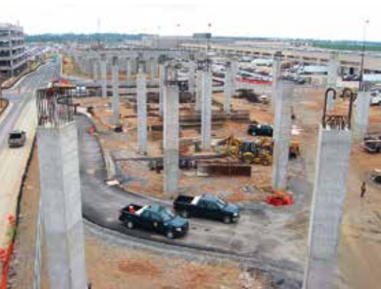
A forest of cast-in-place, reinforced concrete piers rises from the former site of a key Atlanta airport service road. Each pier is supported by spread footings and auger-cast concrete piles.
