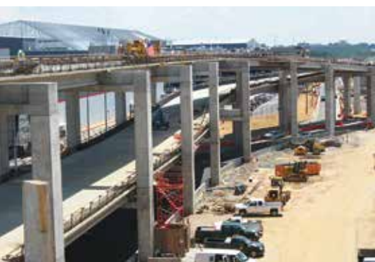
All three levels of the roadway are visible in this view. The ground level is for service access, the second level is for arrivals, and the top level is for departures.
