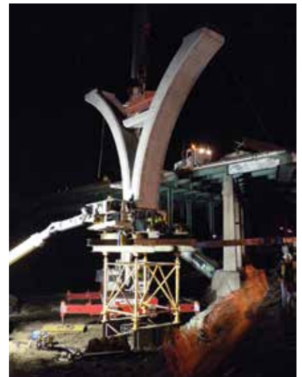
The piers were cast horizontally, rotated, and threaded into the shoring towers.
