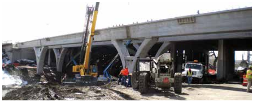
The simple-span girders were spliced and post-tensioned together and connected to the piers and abutments.
