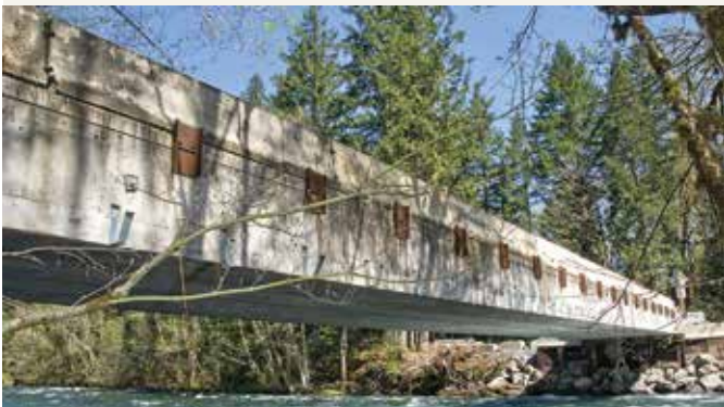
Four 115-ft-long beams from a temporary freeway detour bridge were salvaged to replace a severely load-limited bridge over Oregon’s McKenzie River. All photos: Oregon Department of Transportation.
