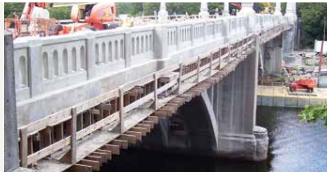
The spandrel arch bridge was restored to its original appearance using modern materials. Photo: American Structurepoint.
