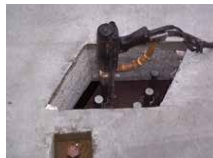
Interstate I-39/90 deck with studs in pockets at 48-in. spacing. Photo: University of Wisconsin.
