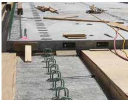
Installed precast concrete deck panels with pockets and beams with shear connectors. Photo: Purcell Associates.
