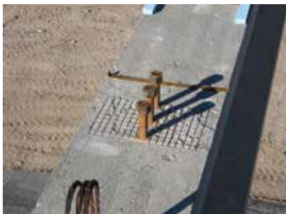
Three threaded-rod shear connectors extending from the girder will be grouted into the blockout in the Texas Department of Transportation deck panel. Photo: TxDOT.
