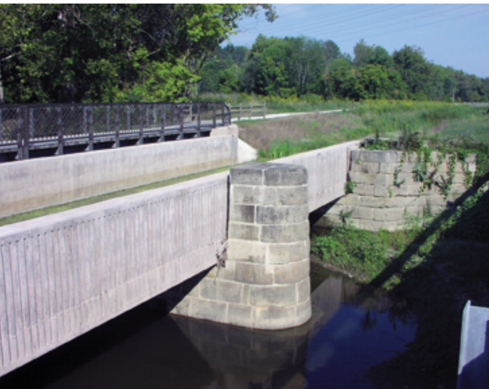
Elevation view of the new aqueduct and fully reconstructed masonry pier. Photo: Henry G. Russell Inc.
