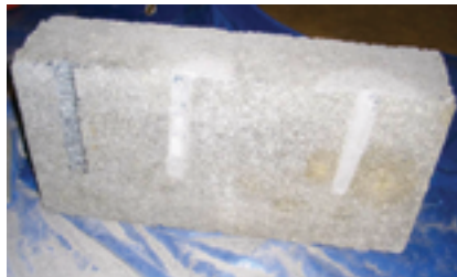
The hole on the left is correctly cleaned. The two holes on the right are still dusty. An epoxy adhesive will not correctly adhere to an improperly cleaned hole.
