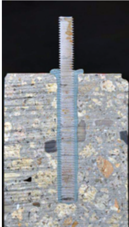
An example of a correctly installed adhesive anchor. All photos: Neal Anderson.
