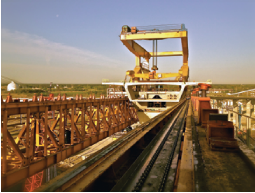
Span-by-span construction techniques were used to build typical spans. Precast concrete segments were delivered across previously built portions of the bridge and placed on triangular trusses, working from the completed bridge.
