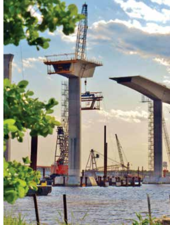
Precast concrete segmental balanced cantilever construction using a barge mounted crane was used to construct the bridge's long main spans over the river.
