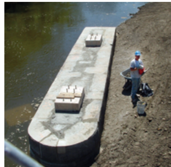
Center pier masonry reconstructed to just below the bottom of the aqueduct trough. Note the two concrete columns cast inside the pier that support the bearings for the new trough. Photo: Bergmann Associates.
