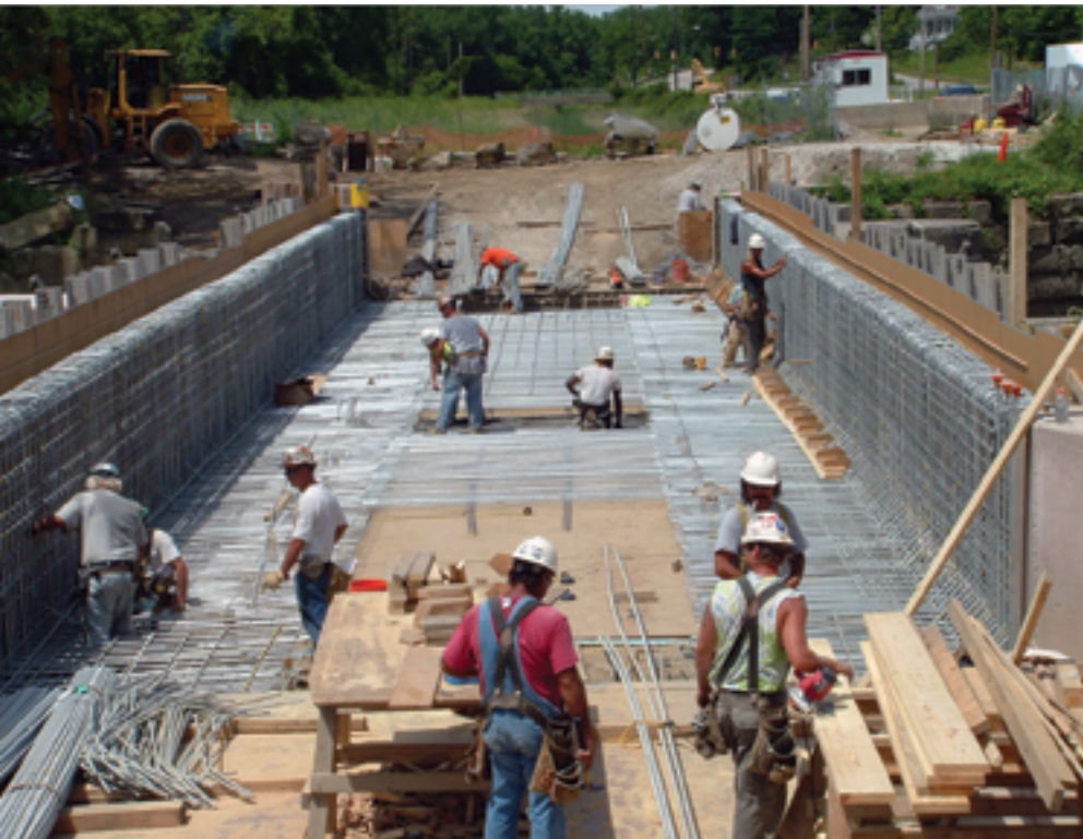
Placement of the galvanized reinforcement for the new trough floor slab and through girder sidewalls. Photo: Bergmann Associates.
