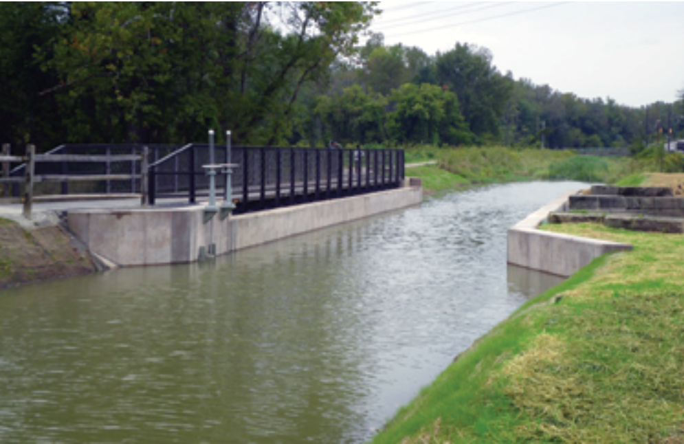
View of the re-watered Ohio & Erie Canal across Tinkers Creek. Manually operated sluice gates in the wall of the transition structure allow for regulation of canal water levels. Photo: Bergmann Associates.
