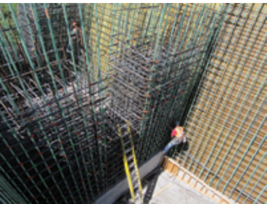
Pier 2 diaphragm, column, and web reinforcing steel, all part of the pier table.
