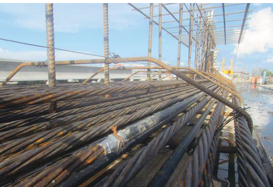
End of debonding tube sealed with duct tape to the strand. Photo: Standard Concrete Products.
