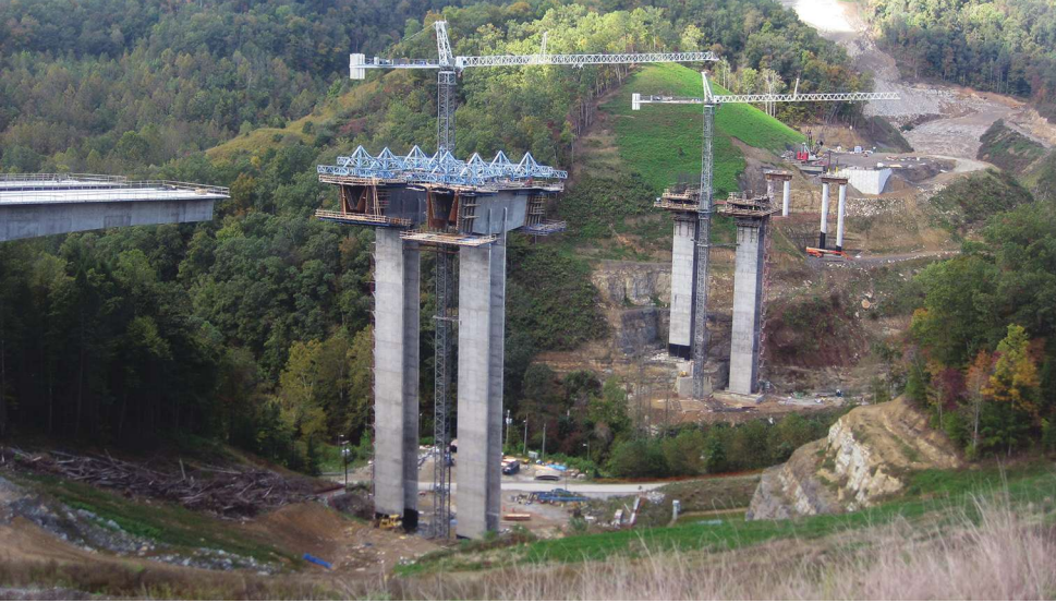
The tallest pier is 261.5 ft tall from bottom of the footing to top of the superstructure.
