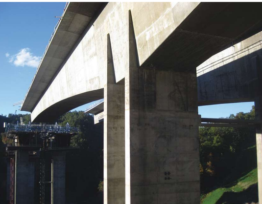
The walls of the H-shaped pier columns continue into the box girder to provide an integral connection.
