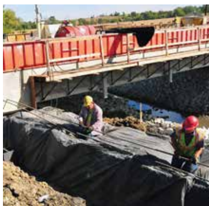
Preparing the high-strength threaded rods to pull the prefabricated bridge superstructure into position.
