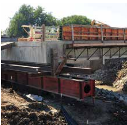
The new bridge superstructure nears completion. A jacking frame has been installed for a test roll.
