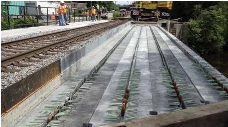
North approach view of the two main tracks looking north on bridge 2 over the Neponset River bridge.
