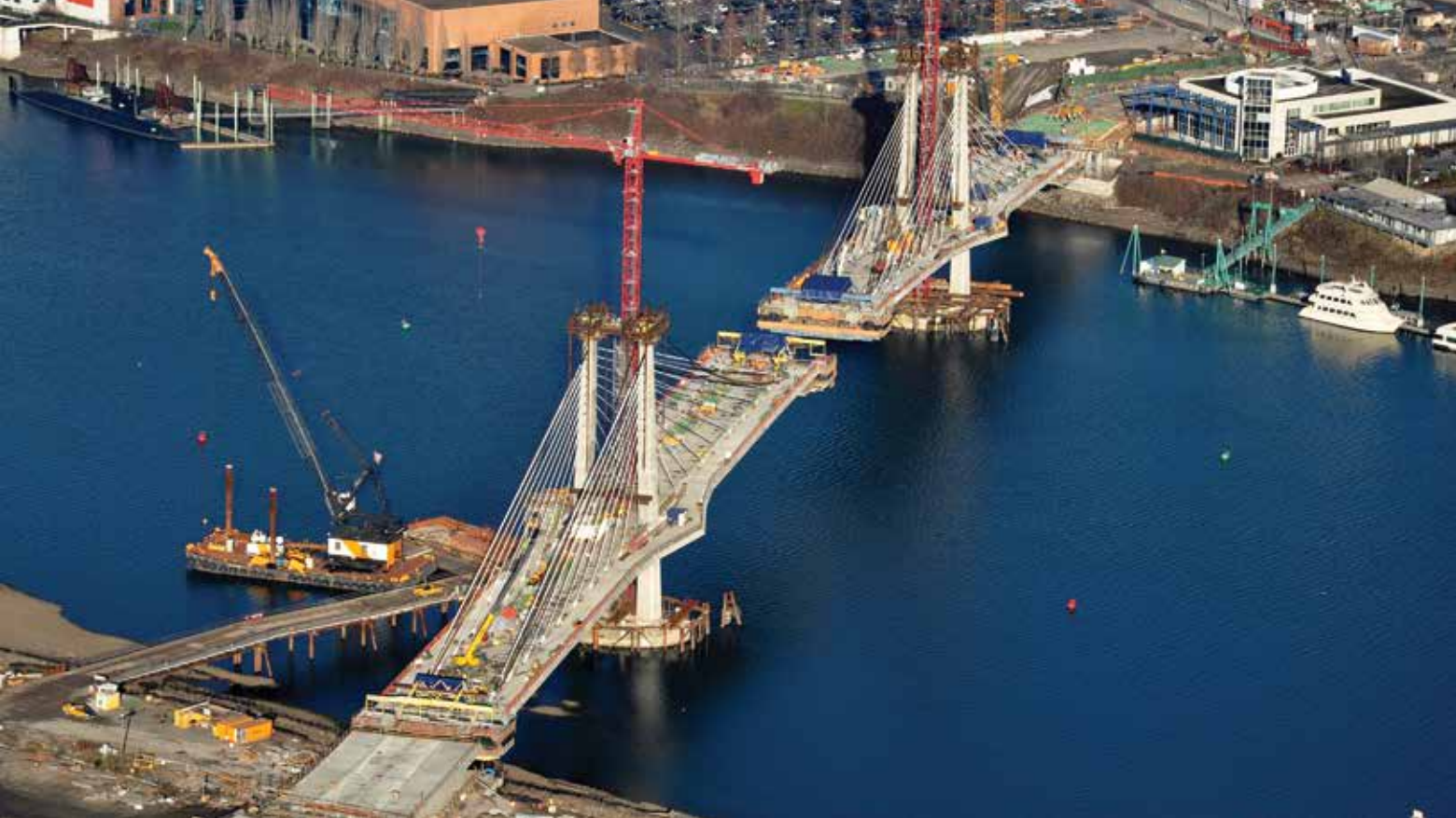
Kiewit combined concrete segmental and cable-stayed technology to design and build the Portland-Milwaukie Light-Rail Transit Bridge for TriMet in the Portland, Ore., metro area.
