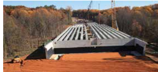
The $550-million, 7-mile-long Intercounty Connector Contract B project in Maryland features 10 precast concrete bridges that had to pass over sensitive stream valleys and two local watersheds.
