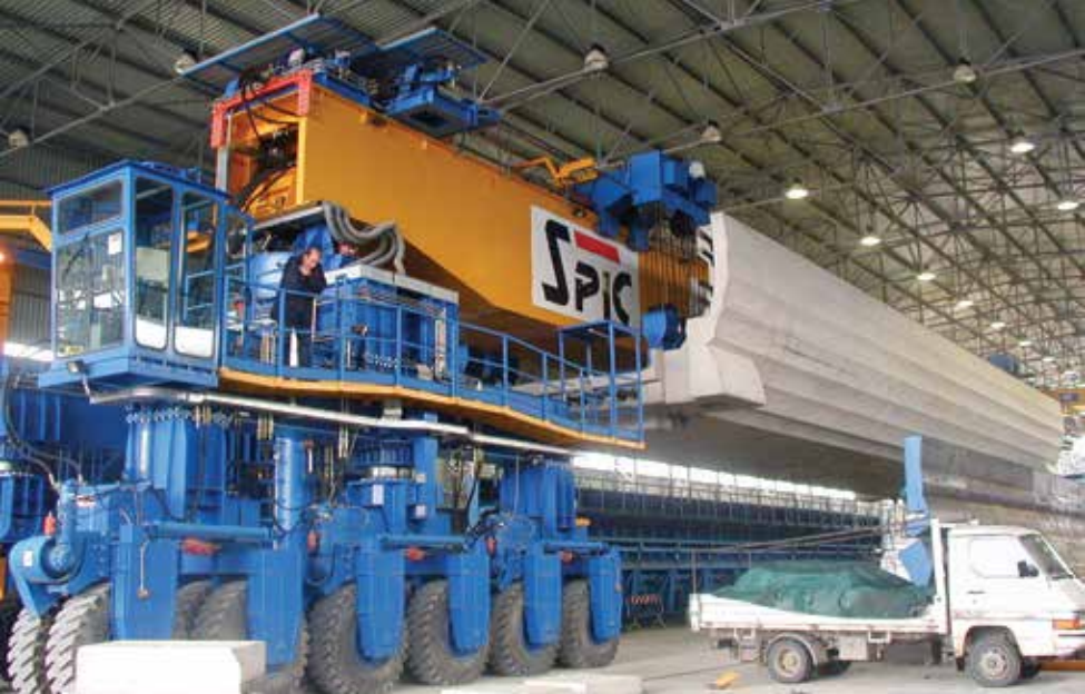
Span transfer to the storage platform with a portal carrier with pivoted tractors. Photo: Marco Rosignoli.
