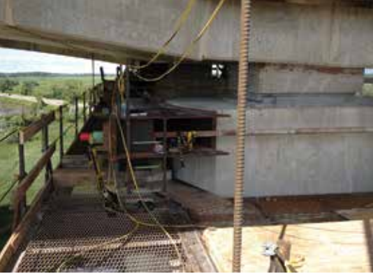
Pier column compression collars.
