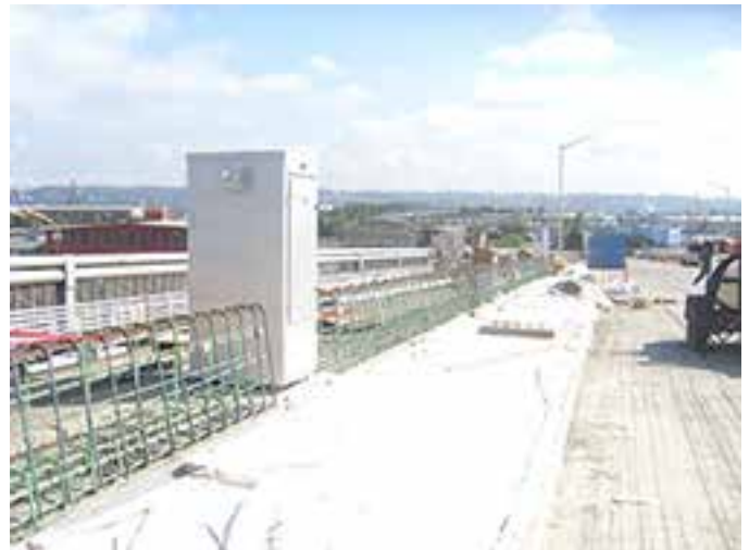
Murray Morgan Bridge port approach looking east— modifications to curbs on deck. Photo: David Evans and Associates Inc.
