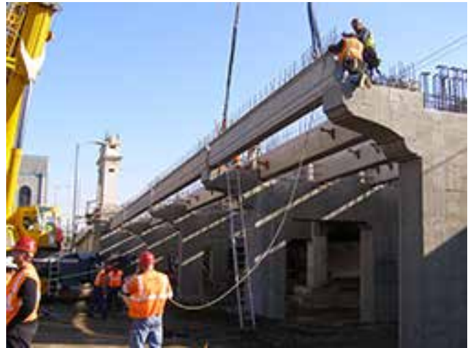
Aesthetic features were formed at the exterior precast concrete girders of the approach spans. Photo: Atkins North America.
