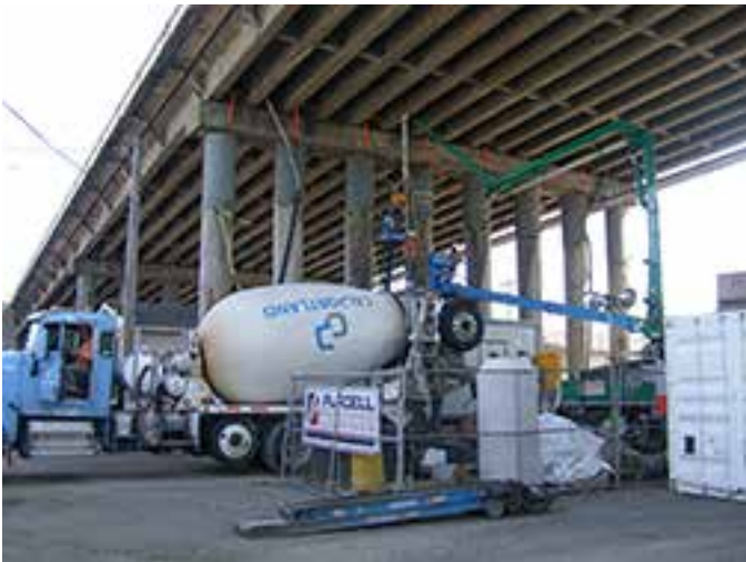
Murray Morgan Bridge port approach looking east—grouting annular space between column and casting. Photo: David Evans and Associates Inc.
